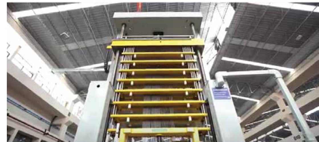
Heat Exchanger Set Up At Air Conditioner Manufacturing Facility, Shirwal, Maharashtra
